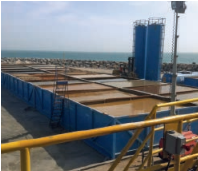
TWMA drill cuttings storage on ZADCO's UZ 750 South Island
