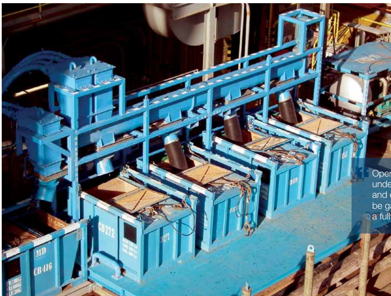
TWMA skip filling station on board the Maersk Discoverer
